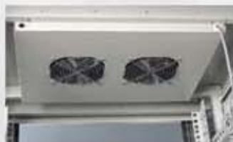
• Cabinets Are Vented To Allow Cooling Fan
