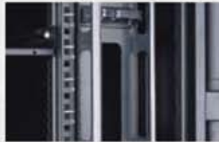
• Cable Management Panels With Cap
